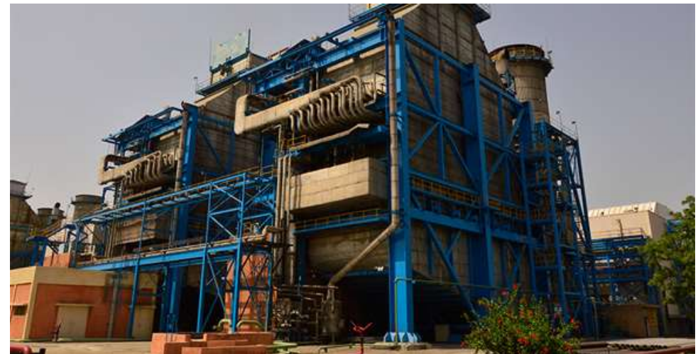
NTPC Dadri Stage II – Unit #6 490 MW
